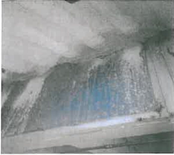
No. 19 – SSV office 192 plenum, water intrusion at sloped roof and original building decking
