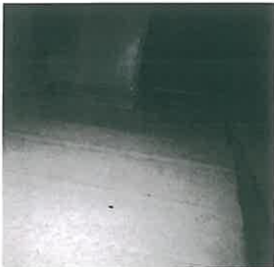
No. 17 – SSV office 192 plenum, rodent droppings
