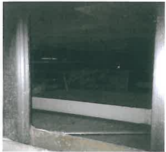
No. 18 – SSV office area 190 plenum, breach in HVAC duct
