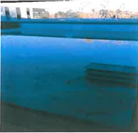
No. 15 – SSV roof with pooled rain water
