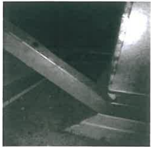
No. 16 – SSV office 192 plenum, debris surrounding supply vent
