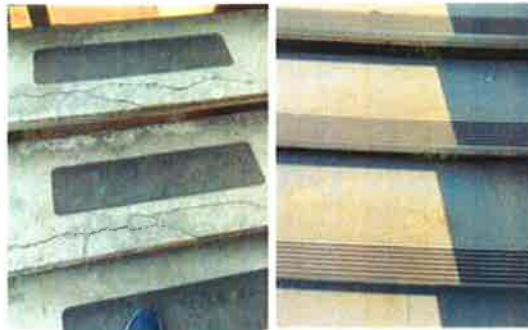
Photo 9 - Damaged stairs front and back
