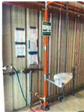
Photo 16 - Emergency Eyewash and Deluge Shower
