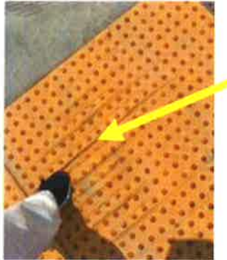
Photo 6 – Damaged Transition Ramp
