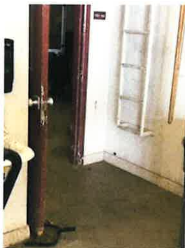
Photo 11 – Trip Fall Hazard
