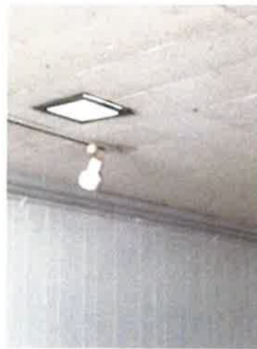
Photo 14 – Loose Ceiling Tiles and Fixture
