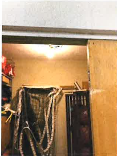
Photo 3 – Exposed Light Bulb
