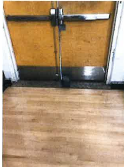
Photo 4 – Trip Fall Hazard
