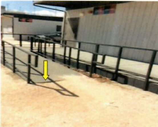
Photo 7 – Trip fall hazard
