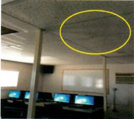
Photo 9 – Stained ceiling tiles
